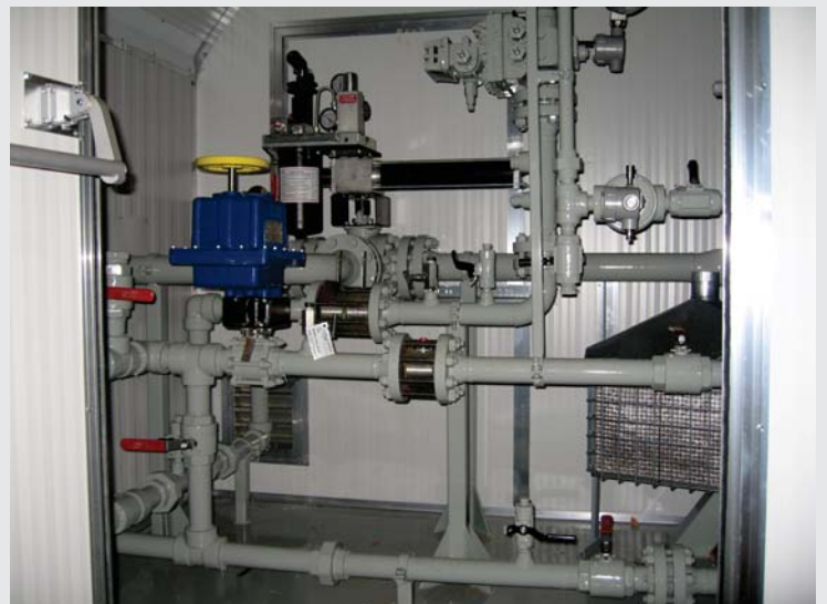
All Electric Control System
